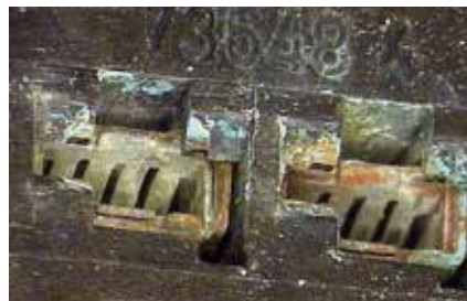
Coupling with traces of moisture and corrosion
